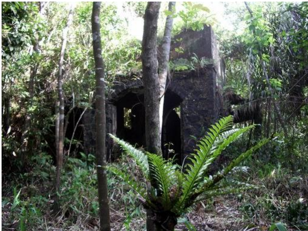
Figure C- 94 SR HS11, Thua Thien Residence, apparently a garage with further accommodation above
