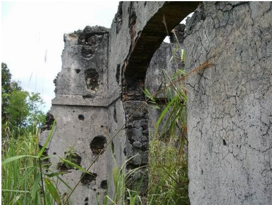
Figure C- 83 WR HS4, Lot 76. Note damage in walls from gunfire.
