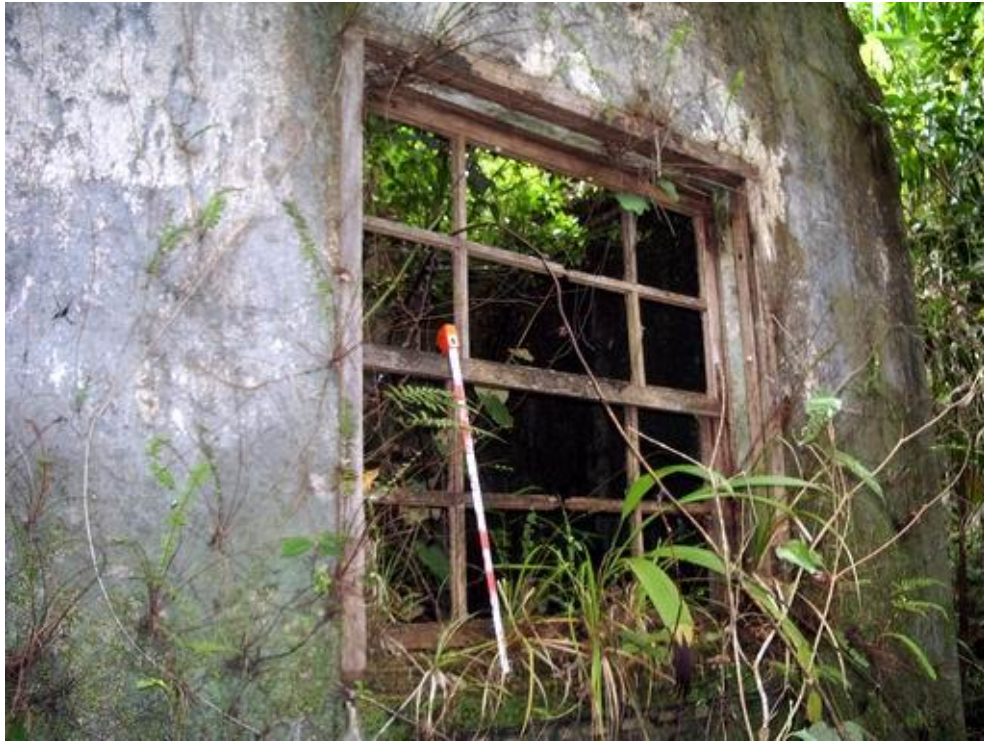
Figure C- 89 - 40 SR HS3, No name. Several structures in the southern zone retained some window and door frames
