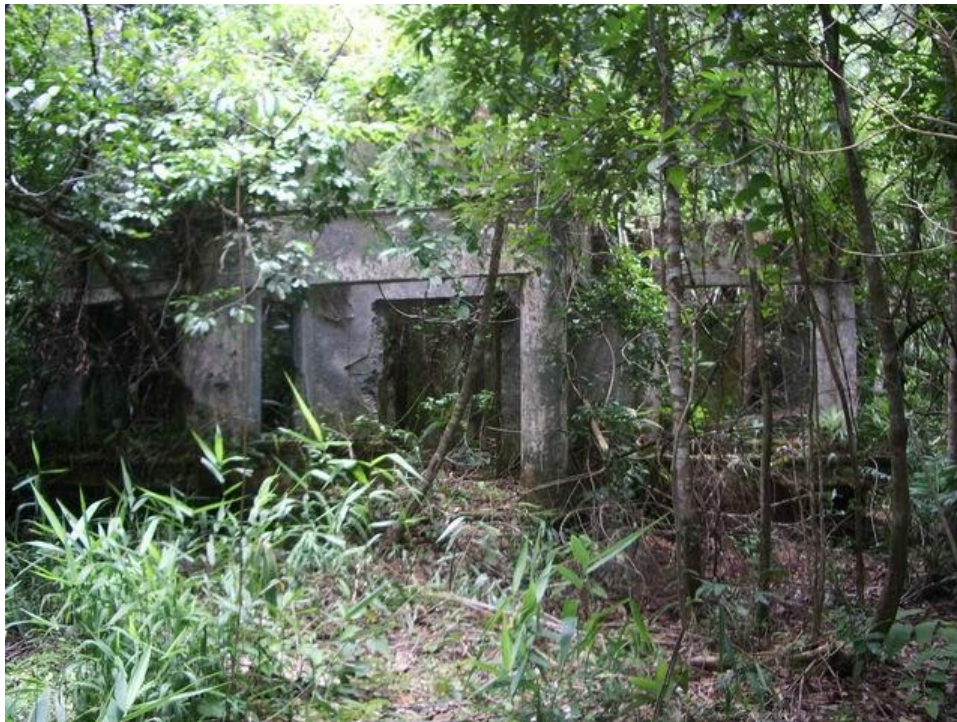
Figure C- 91 SR HS8, Sogny. Note the column marking the entry onto a covered verandah. To the right is a large window looking out from the main living room.
