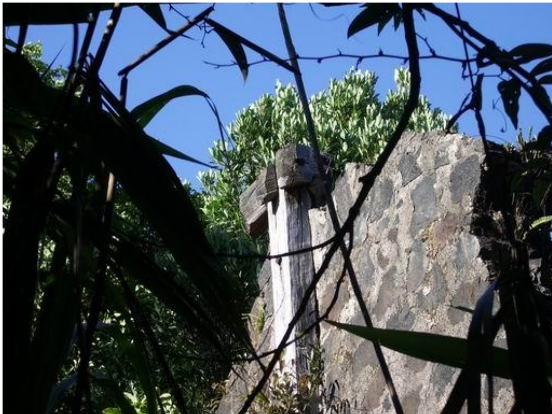
Figure C- 76 CR HS12, Thân Trọng Khôi, the roof beams have been cut for removal
