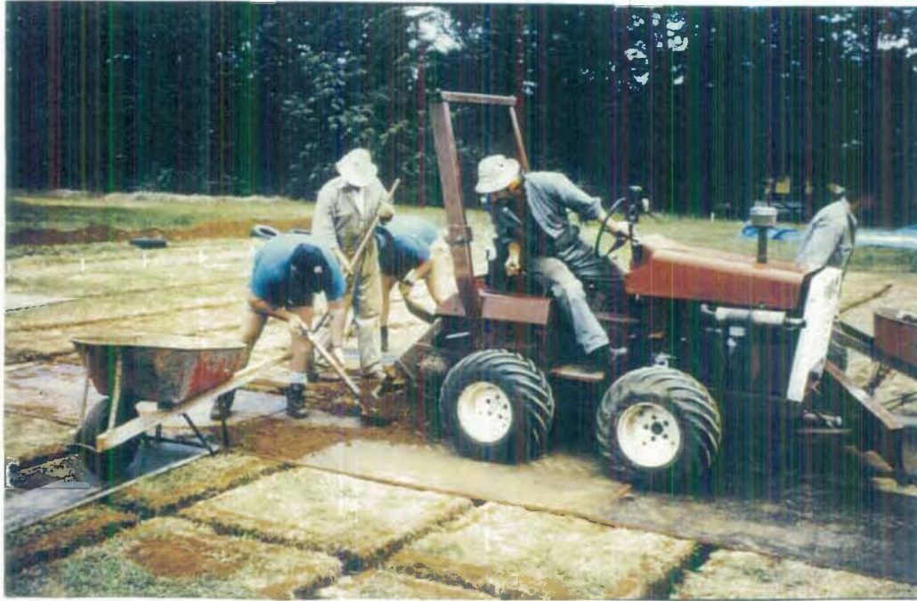
Plate 3.1: A trench digger was used to excavate to 100 cm, around 1 m 2 plots. The digger sat on thick plywood to help prevent soil compaction.
