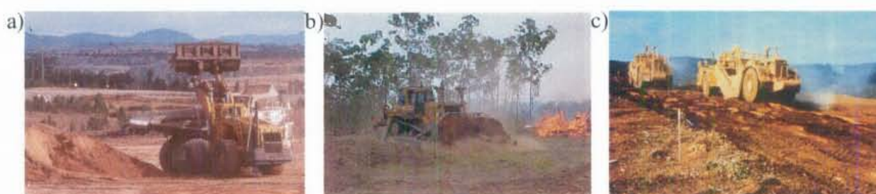
Figure 3.2: Machinery used for the construction of stockpiles (a) loader and truck, (b) bulldozer and (c) scrapers.
