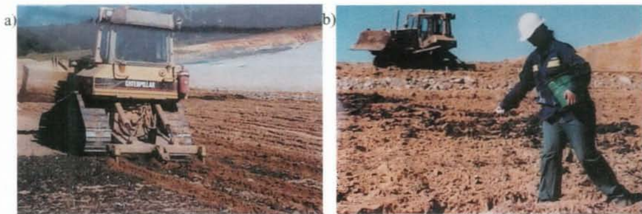
Figure 7.8: (a) Ripping of the area and (b) seeding of the rehabilitation area at Cheshunt mine.
