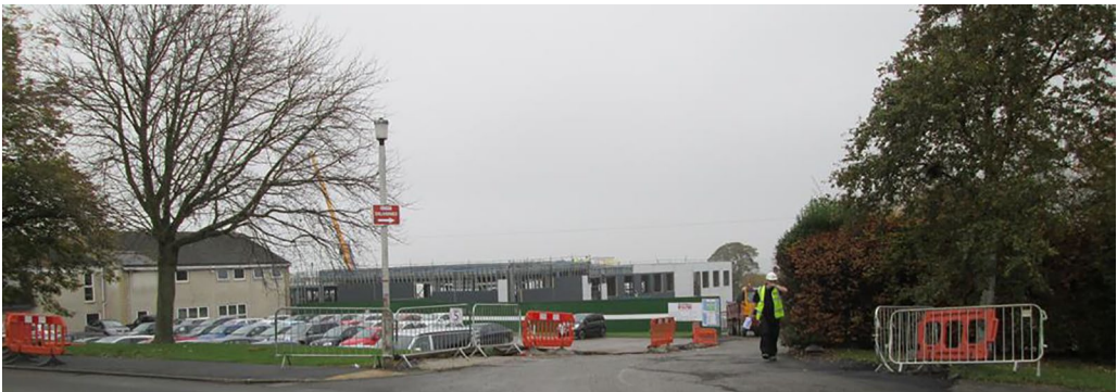
Figure 1. Part of the old school premises (left) with the new building under construction.
