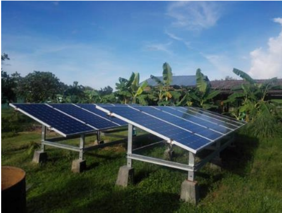
Figure 6-12 Solar Panels on the Farm, September 2015 (source: Ko Than Shwe)
