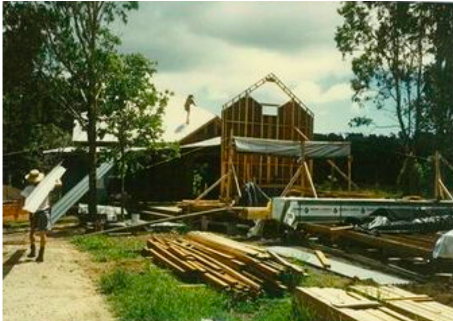
Stage 1 of the Shearwater Building Program in the process of construction, 1995. (Photo: Shearwater archive)
