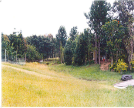
CREEK BED DEPRESSION
