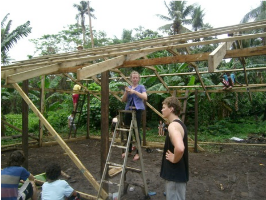
Shearwater students constructing the frame for the Kindergarten building on the village of Laonamoa. (Photo: G Braithwaite, Shearwater archive)
